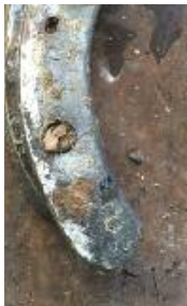
Load and wear again appears to indicate a tight fit. What conditions justify this fit?
